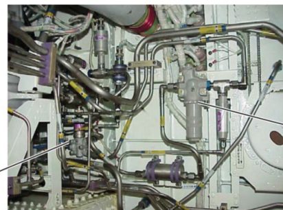
Aux System Components
