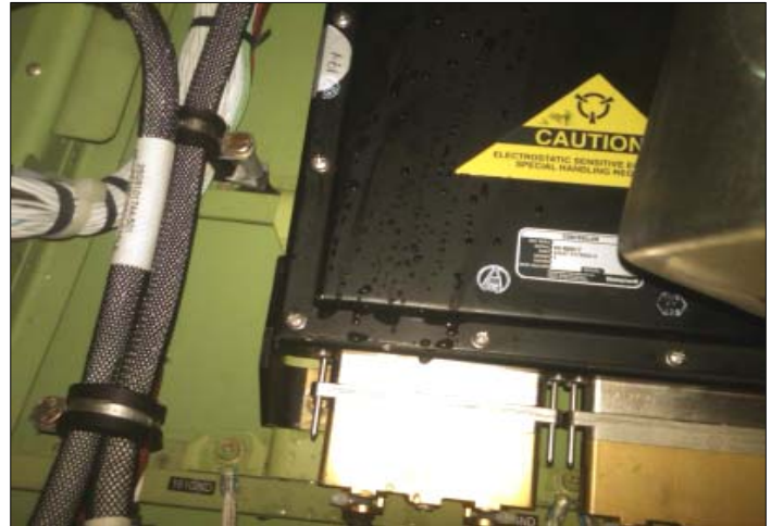
Water on the ECU entered the tail compartment through the APU air inlet.
